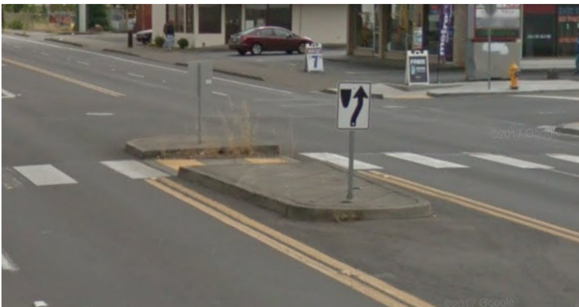
Figure 22. Existing pedestrian refuge island at Fairmount Avenue; Image courtesy of Google Earth
