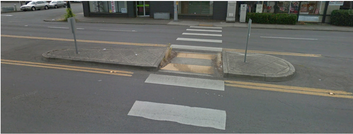
Figure 21. Existing pedestrian refuge island at Z Street; Image courtesy of Google Earth
