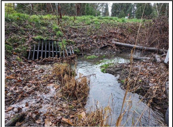
Outfall monitoring station CSL1 – 1/9/2024
