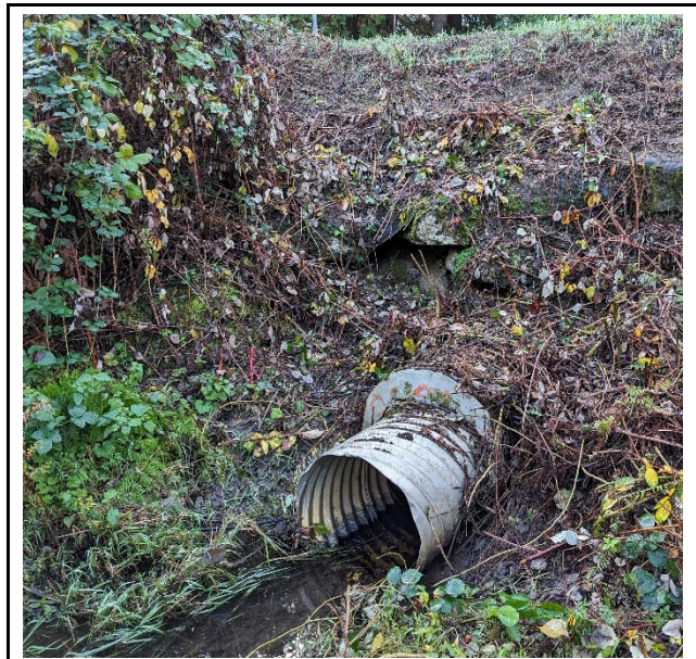
Outfall monitoring station CSO1 – 10/18/2023
